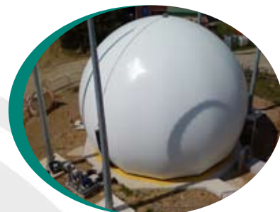
Sewage Treatment Works for Thames Water - Bishop Stortford
